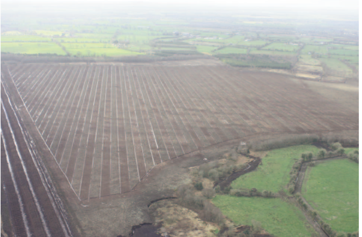
Figure 2: Air photograph looking south showing the extent of the drainage works undertaken on Clonroosk Little Bog, Cos Kildare and Offaly some time between October 2013 and March 2014.
